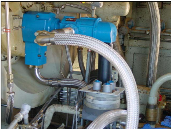
Figure 7. Air Starter Installation
